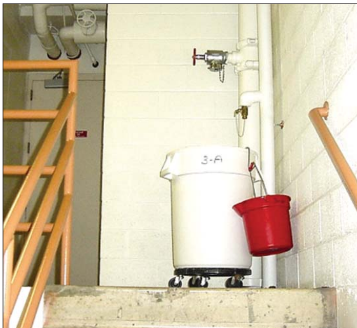
At Inova Mount Vernon Hospital in Alexandria, Va., emergency water carts are stationed at the stairwell standpipe to supply water for manual toilet flushing and other uses.
