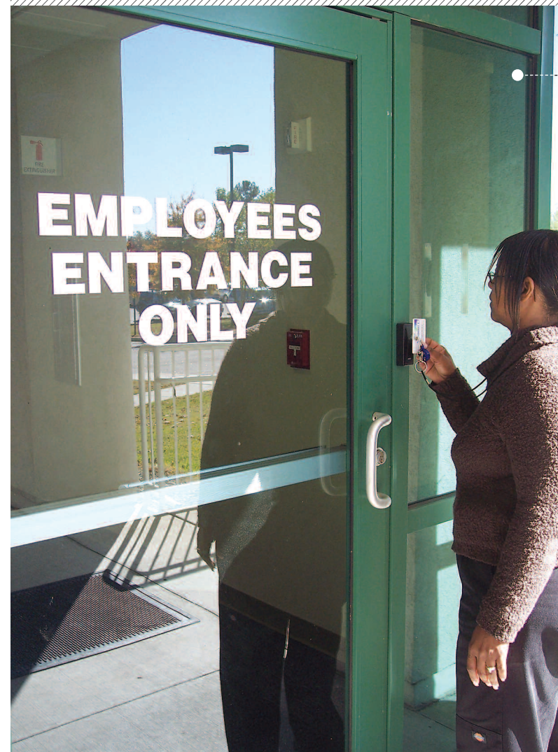
SAFE APPROXIMATION Sandhills Regional Medical Center in Hamlet, N.C., uses Schlage wireless proximity card readers in tandem with a Schlage web-enabled security system to access, monitor and manage its system from any computer running a standard web browser. Ingersoll Rand Security Technologies
