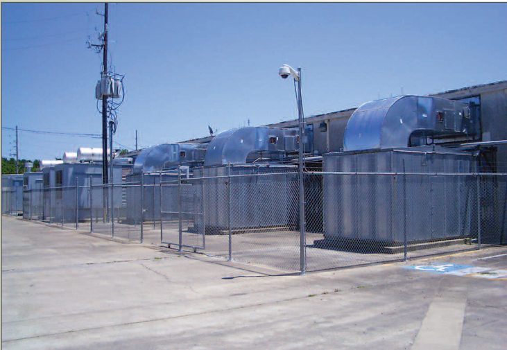
A fence and a video camera in plain sight deter unauthorized access to this arrangement of three generators in the background and three mechanical air handling units in the foreground.
