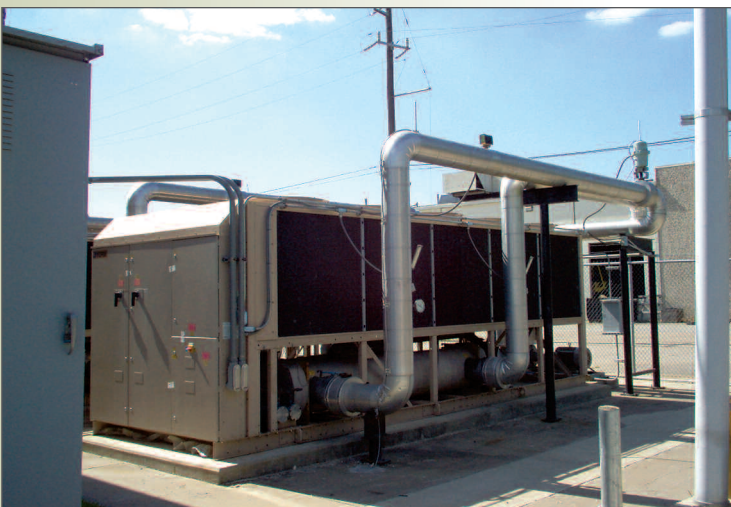
A slab-mounted air-cooled chiller supplies chilled water to interior air handling units, while a redundant chiller stands ready in the background.
